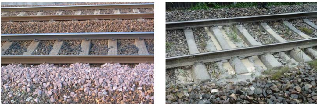
Figure 12. Normal Ballast (left). Loose Ballast (right) Can Create Safety Issues for Trains.
